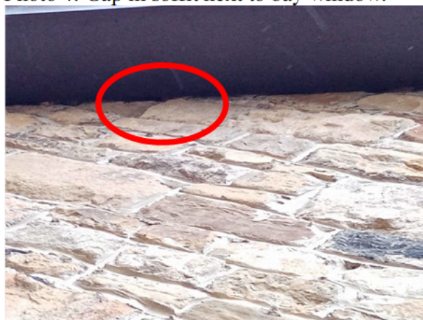
Photo 6: One of a number of gaps present between the soffit and house wall on the west aspect.
