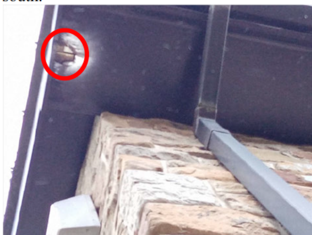
Photo 3: Hole in the underside of the soffit.
