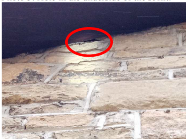
Photo 5: One of a number of gaps present between the soffit and garage gable wall.
