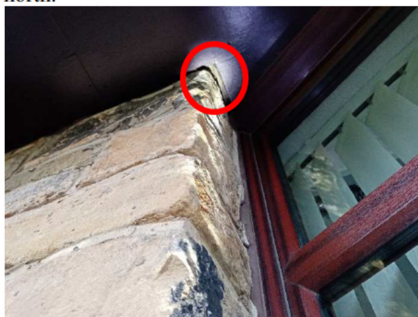
Photo 4: Gap in soffit next to bay window.
