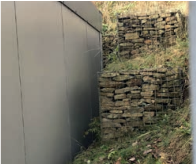
8: View showing the retaining wall elements or gabions for the temporary classrooms.
