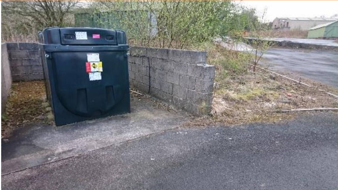
PLATE 6: ABOVE GROUND STORAGE TANK
