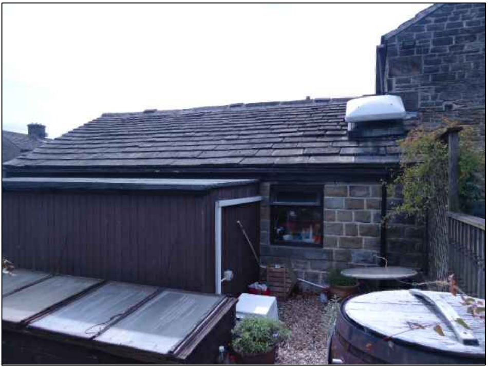
EXISTING PHOTO: EXISTING KITCHEN EXTRACT COWL
