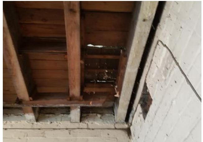
Photo 14: Visible daylight through roof of building 3.
