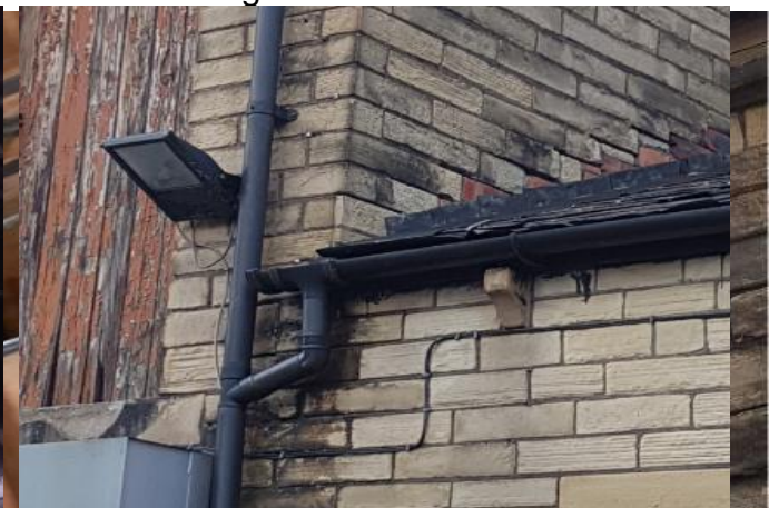
Photo 12: Lifted roof tiles at eaves of building 3.
