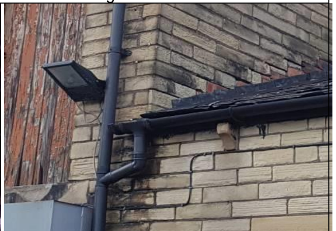
Photo 12: Lifted roof tiles at eaves of building 3.
