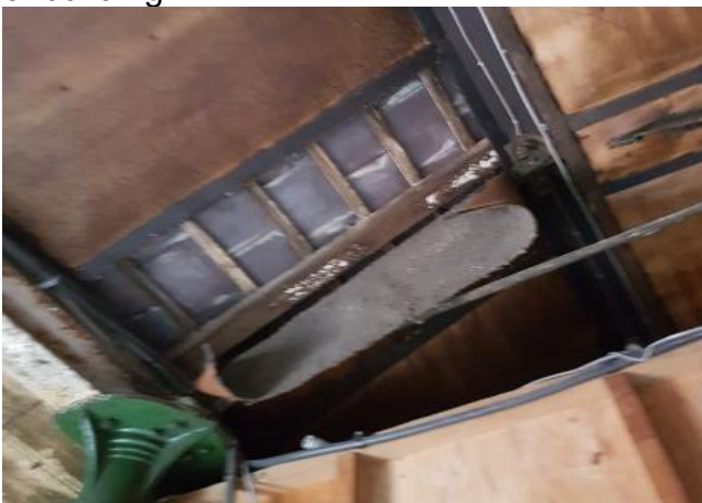
Photo 17: falling insulation tiles and roof visible in building 4.
