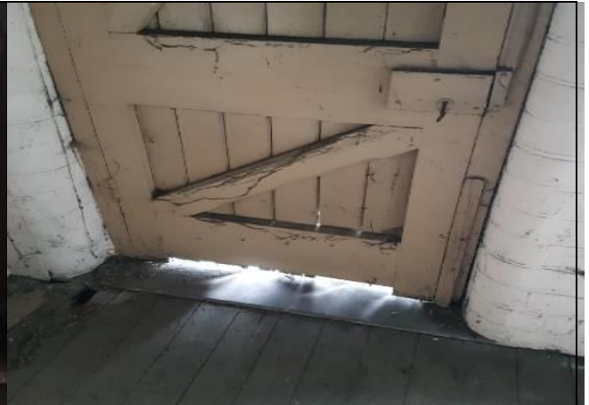
Photo 8: Gap under external door in building 2.
