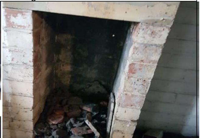
Photo 10: Open chimney breast on second floor of building 2.
