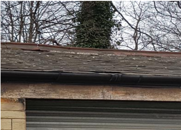
Photo 13: Lifted ridge tiles on building 3.
