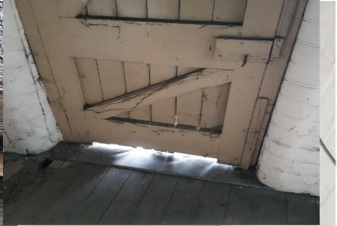
Photo 8: Gap under external door in building 2.
