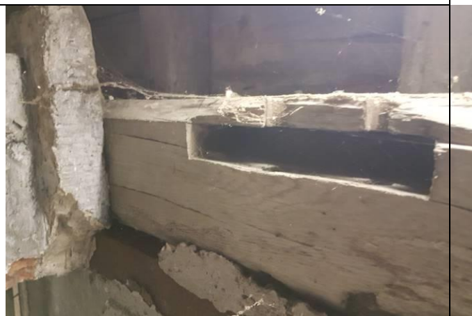
Photo 4: Cavity within timbers in cellar of building 1.
