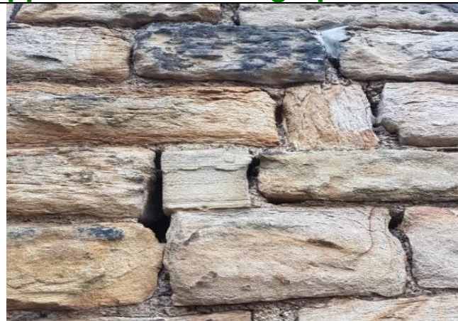
Photo 1: Missing/damaged pointing on building 1.
