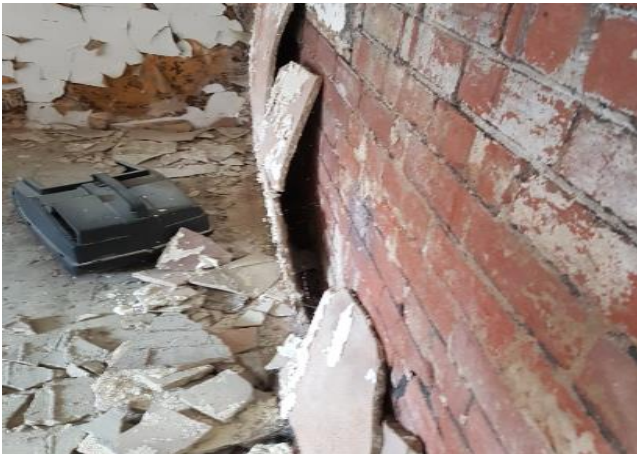
Photo 15: Void created behind plasterboard of building 4.
