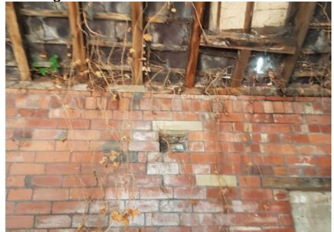
Photo 16: Airbrick and visible daylight in building 4.
