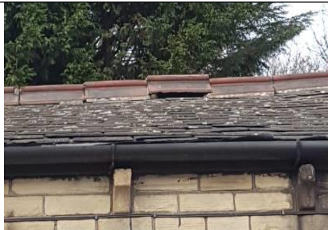
Photo 2: Lifted tile along the roof ridge and at the eaves of the roof.
