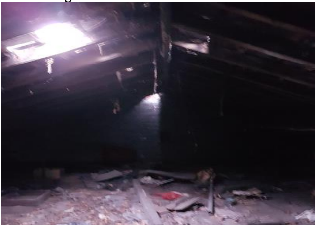
Photo 11: Roof in state of collapse with gaps evident in building 2.
