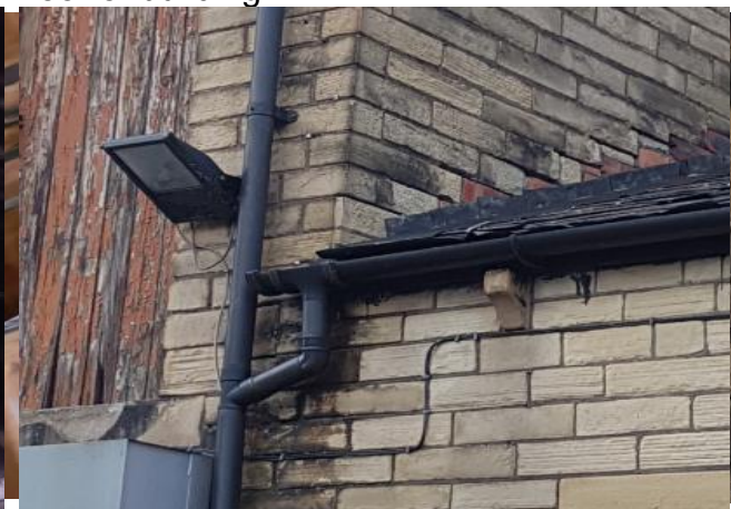
Photo 12: Lifted roof tiles at eaves of building 3.
