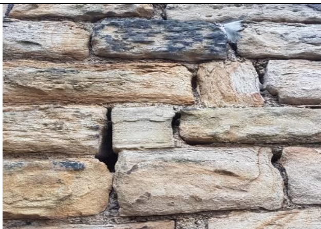
Photo 1: Missing/damaged pointing on building 1.
