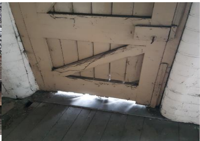
Photo 8: Gap under external door in building 2.
