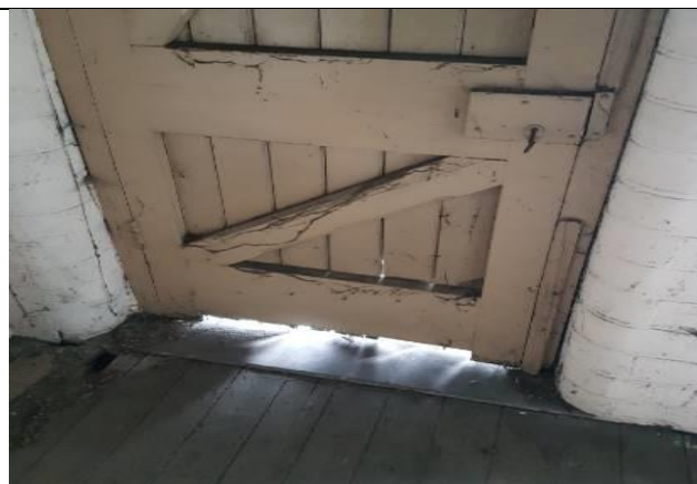
Photo 8: Gap under external door in building 2.
