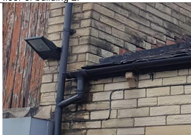
Photo 12: Lifted roof tiles at eaves of building 3.
