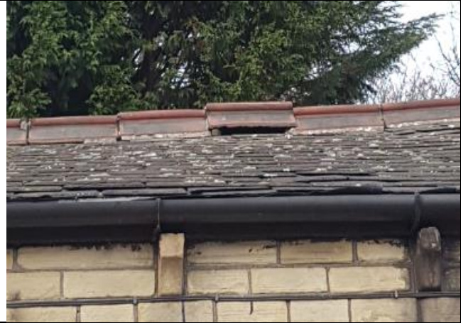
Photo 2: Lifted tile along the roof ridge and at the eaves of the roof.
