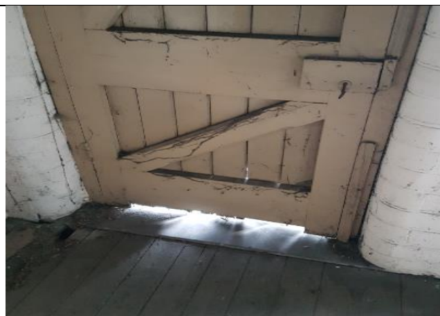
Photo 8: Gap under external door in building 2.
