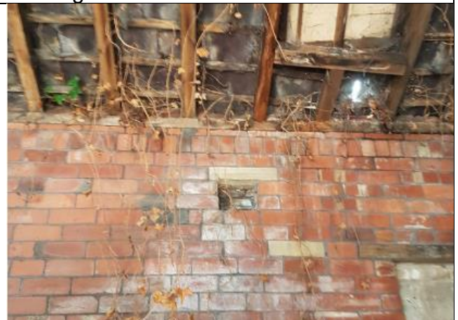
Photo 16: Airbrick and visible daylight in building 4.
