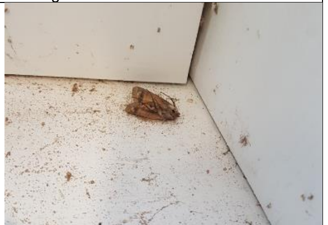
Photo 6: Intact moth within building 1.
