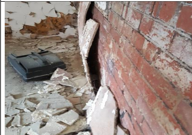
Photo 15: Void created behind plasterboard of building 4.
