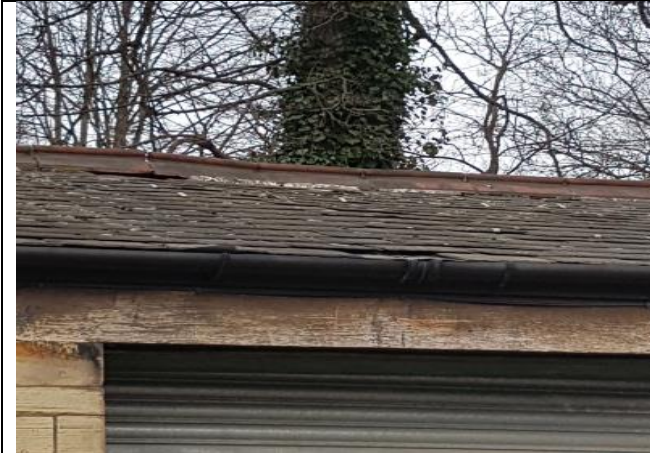
Photo 13: Lifted ridge tiles on building 3.
