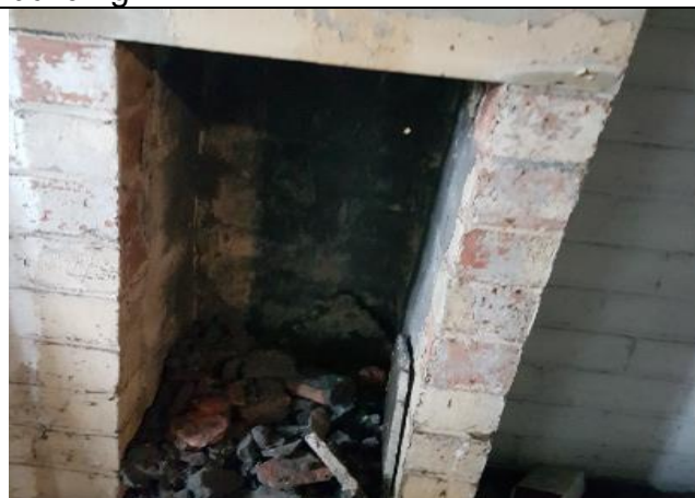
Photo 10: Open chimney breast on second floor of building 2.
