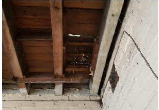
Photo 14: Visible daylight through roof of building 3.
