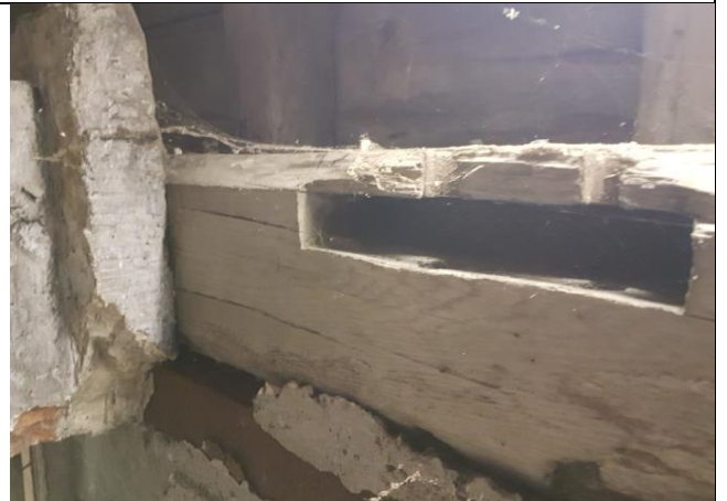
Photo 4: Cavity within timbers in cellar of building 1.
