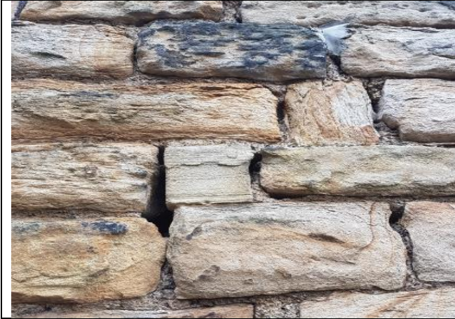
Photo 1: Missing/damaged pointing on building 1.
