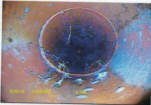
, 00:01:13, 0.70 m Roots, tap at joint
