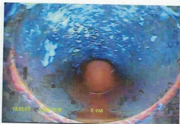
, 00:00:13, 0.01 m Joint displaced, medium
