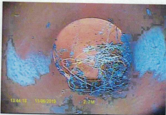
, 00:00:44, 2.70 m Roots, mass at joint, 40% cross-sectional area loss
