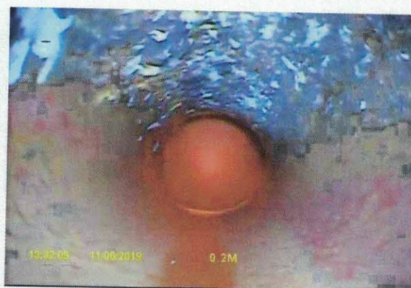
, 00:00:14, 0.20 m Attached deposits, fouling from 10 o'clock to 2 o'clock, 10% cross-sectional area loss
