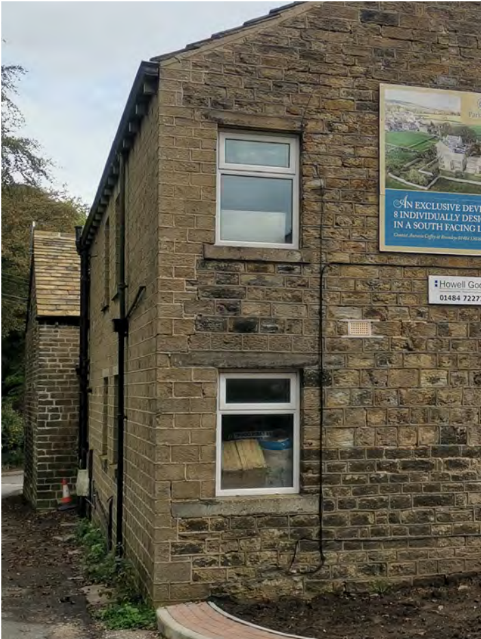
IMAGE 9_ SHOWING NEW STONEMWORK TO NORTH FACADE BEING POORLY TIED IN TO WEST GABLE.
