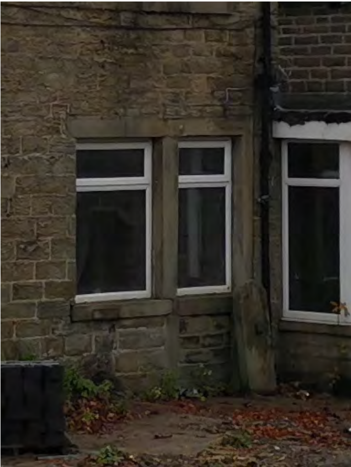
IMAGE 11_ IMAGE SHOWING NEW STONE ON NORTH FACADE BEING POORLY TIED IN TO WEST GABLE.
