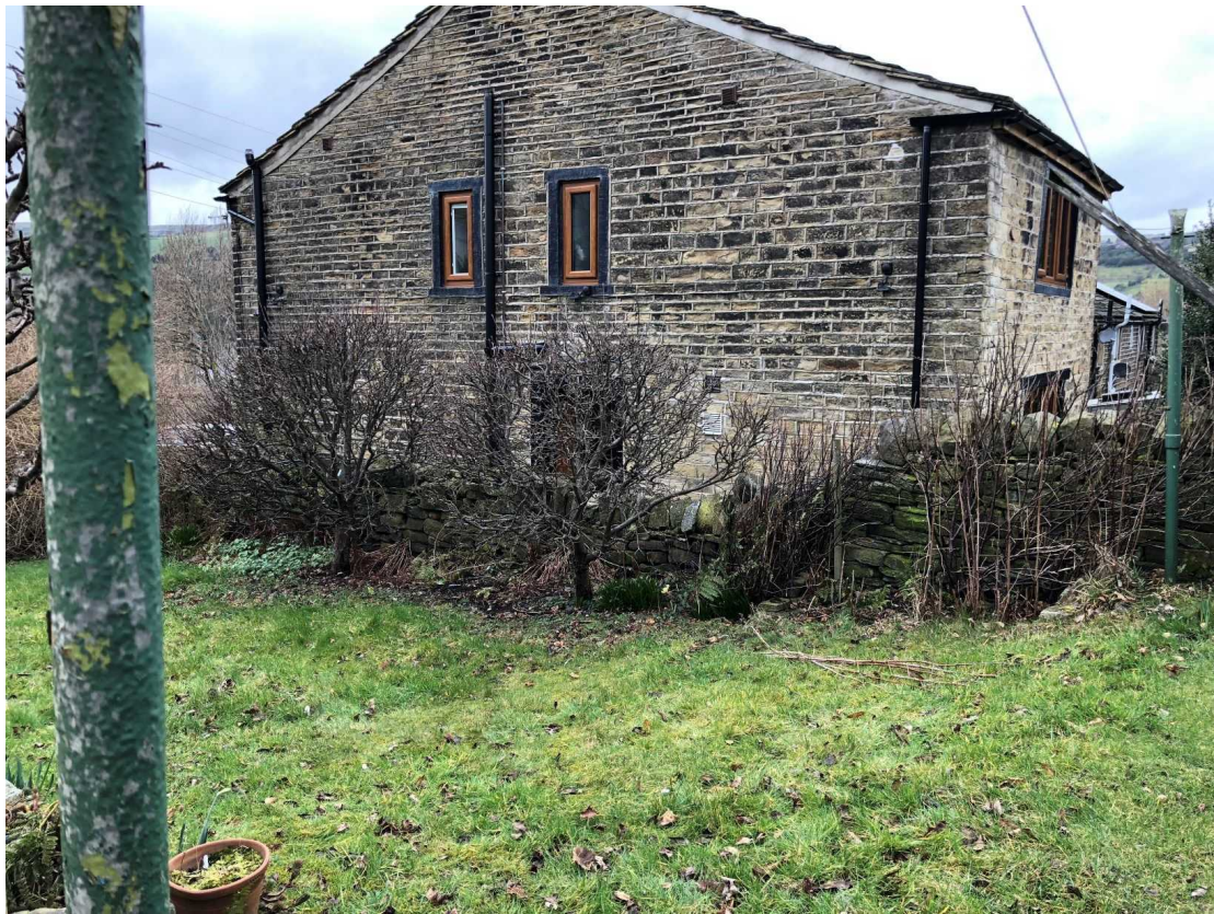
Image 2 - No.33 Gable with Non Habitable Windows
