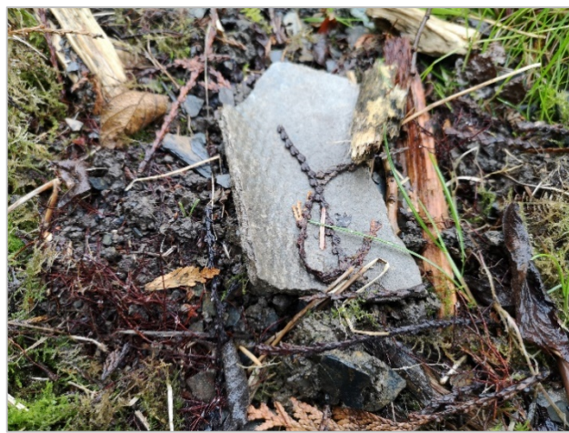
Figure 10 Suspected Asbestos Cement Sheetting
