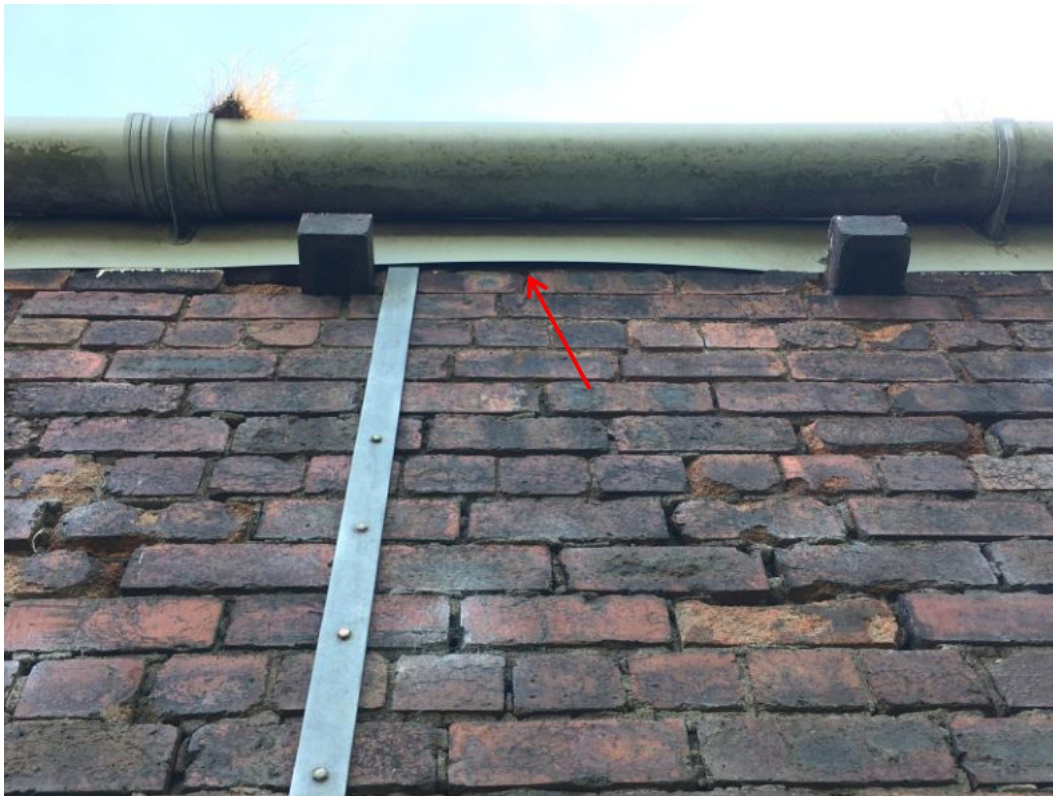
Photo 8. Potential bat roost feature behind eaves cladding on western elevation
