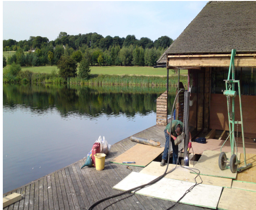
Restricted site working on decking over a lake to provide foundations (Grundomat is inside the casing)
