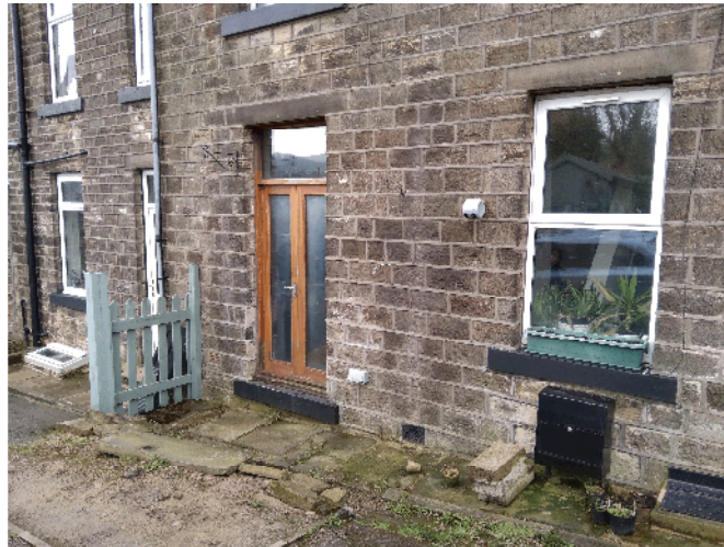
Closer view of location for proposed porch showing the current entrance on the left
