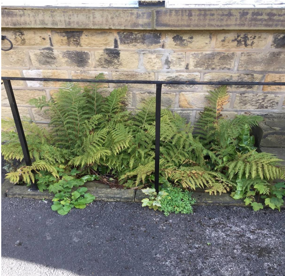
Blocked up basement windows, to be reinstated.
