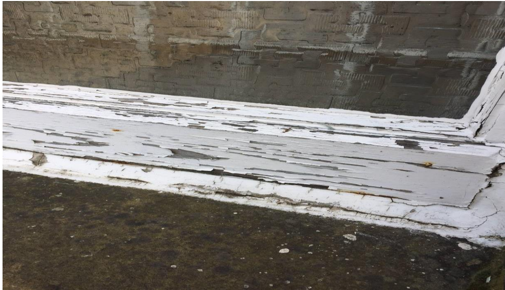
Timber sash windows in disrepair. To be refurbished and conserved.
