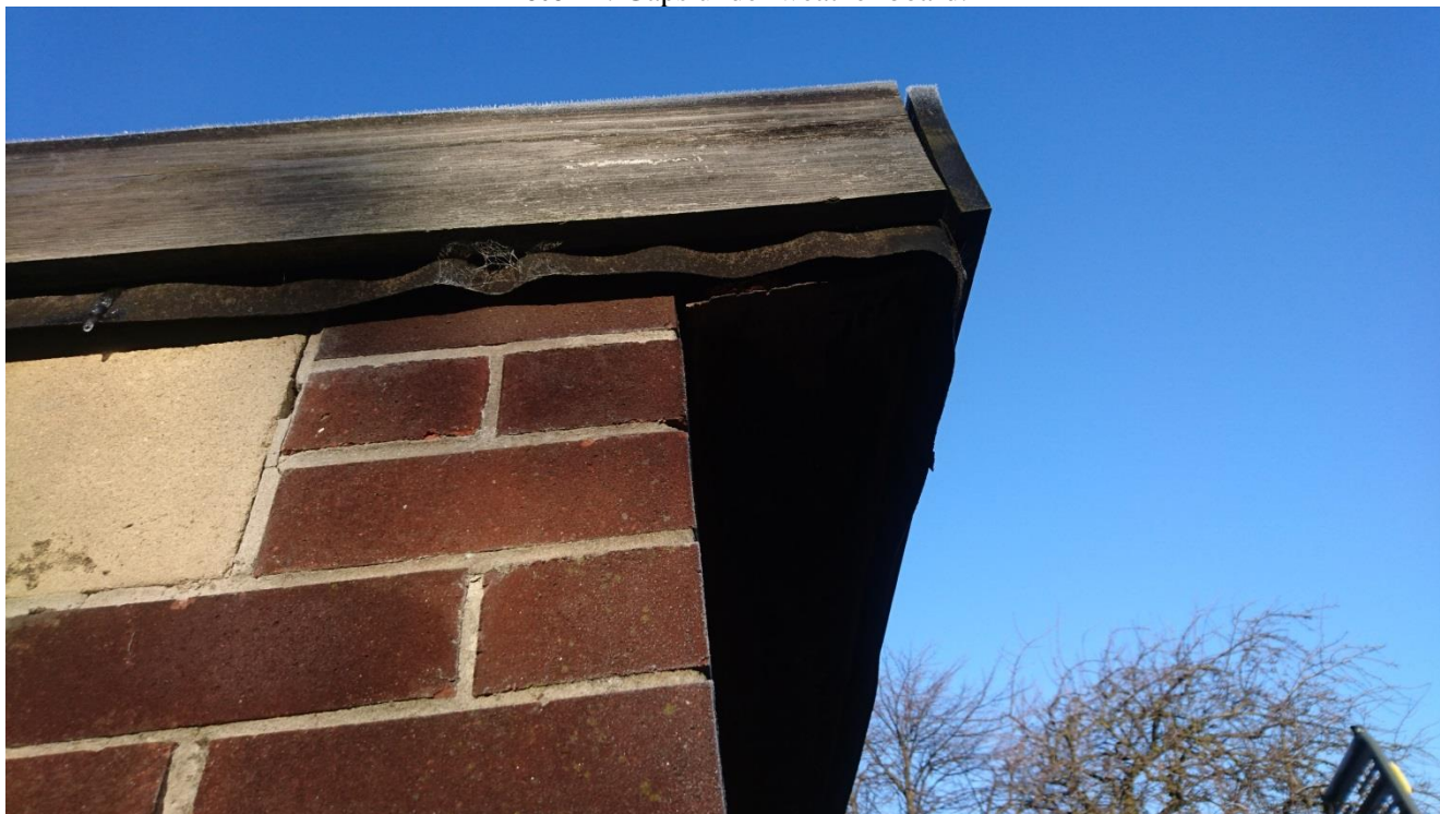
Photo 11: Gaps under weather board.
