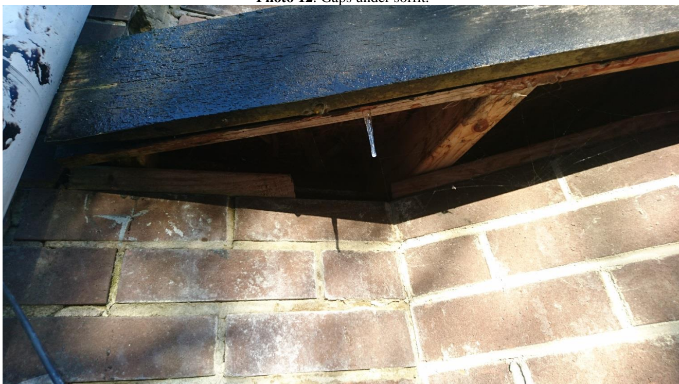
Photo 12: Gaps under soffit.
