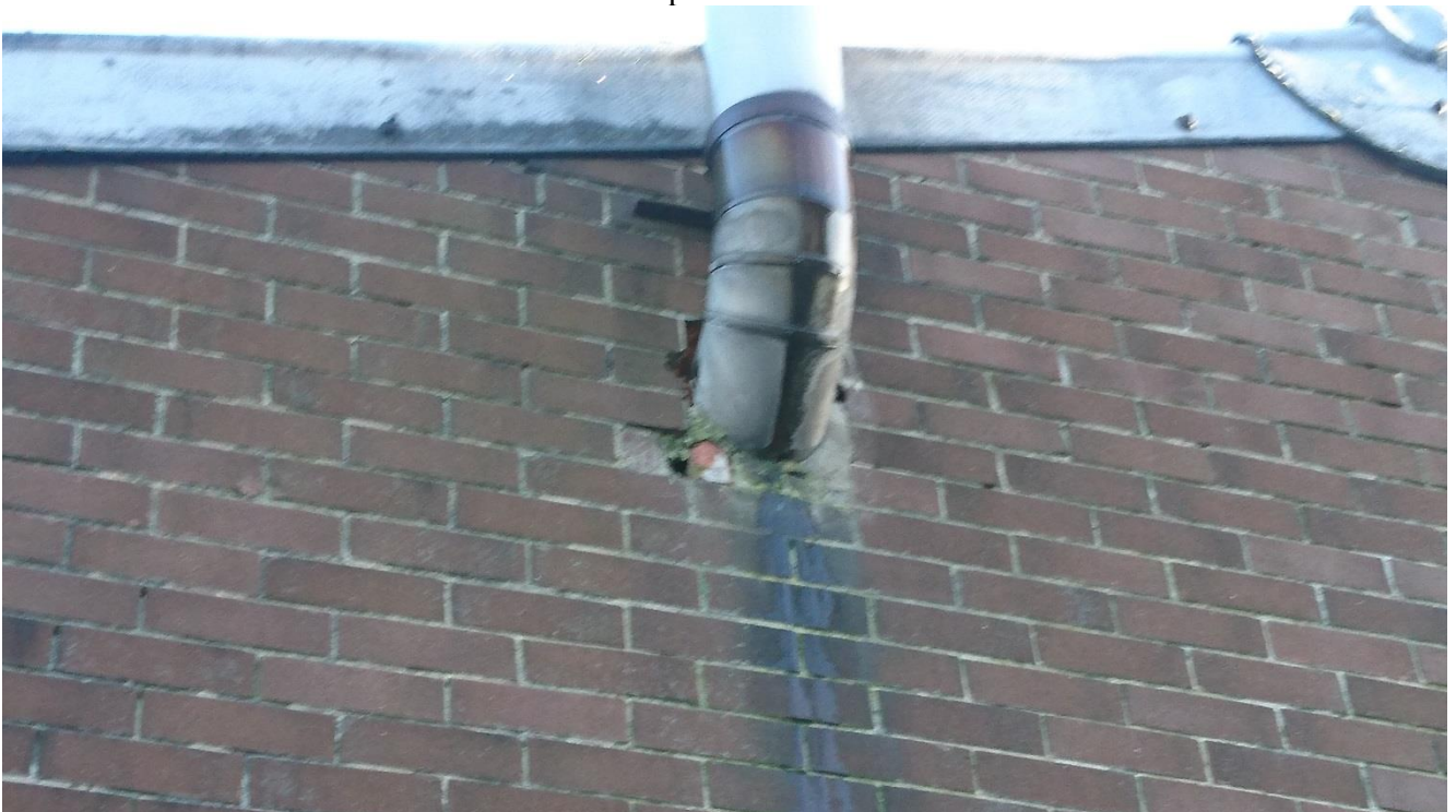
Photo 14: Gaps in brick below flue.
