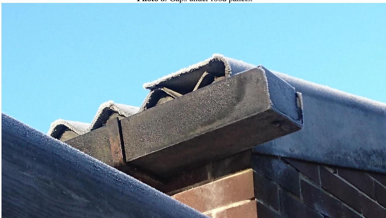
Photo 8: Gaps under rood panels.
