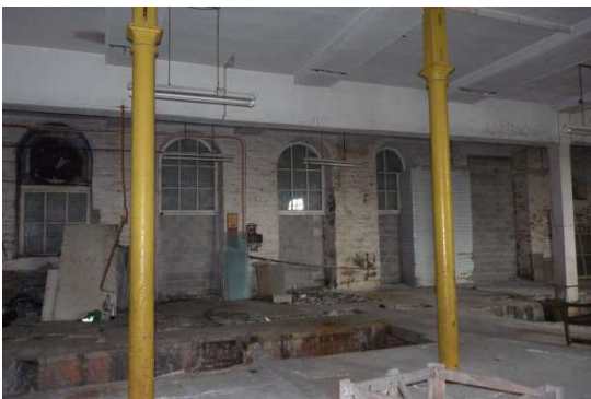
Ducts in the floor
