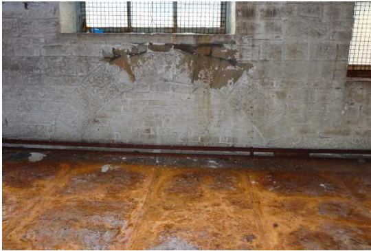
Rust staining on the floor; note an infilled arch below the window
