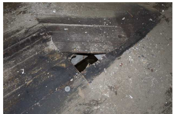
Hole through the floor
