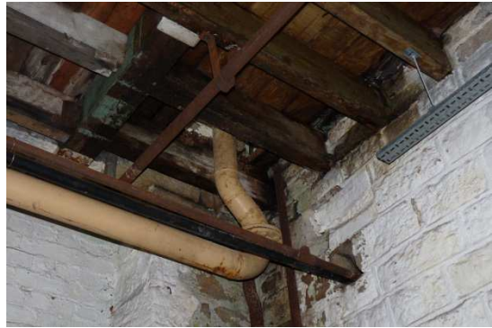
Water ingress through a floor opening
