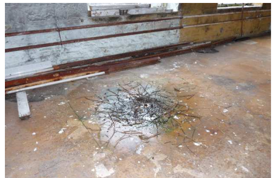
Water and twigs on the floor under the leak
