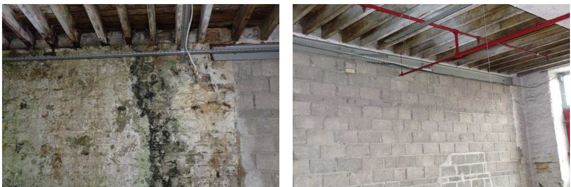
North Gable: water ingress and damp on the existing wall and part re-built wall
