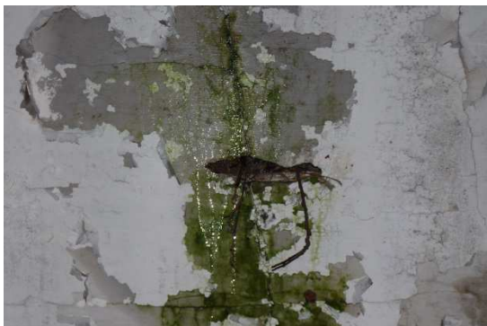
Birds in the roof and leak
