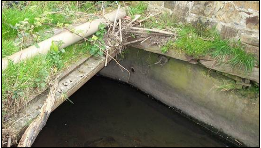
Figure 2: Entry to Hunsworth Beck box culvert through the centre of the site
