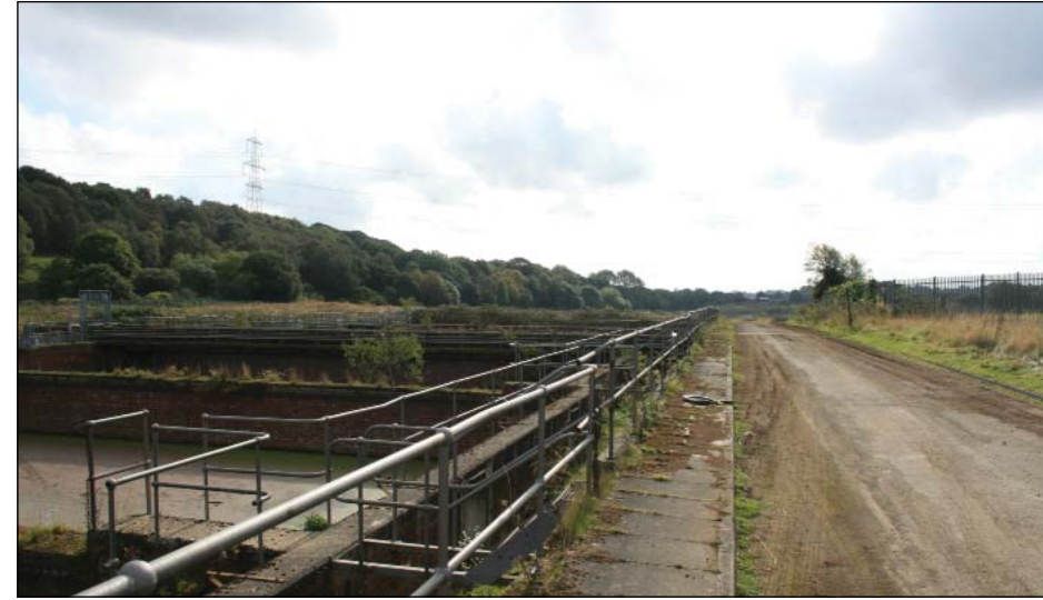
Plate A7.23: Settlement Tanks
