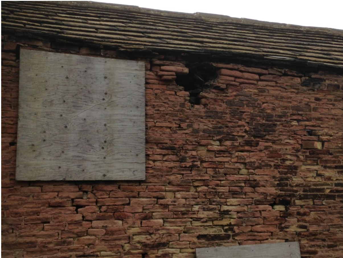
Figure 12- Existing reddened bricks at Poplar Farm
