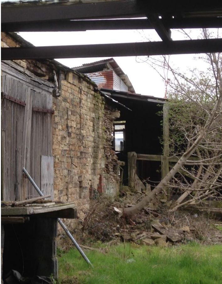
Figure 2- Crumbling farm roof & wall structure at Poplar Farm
