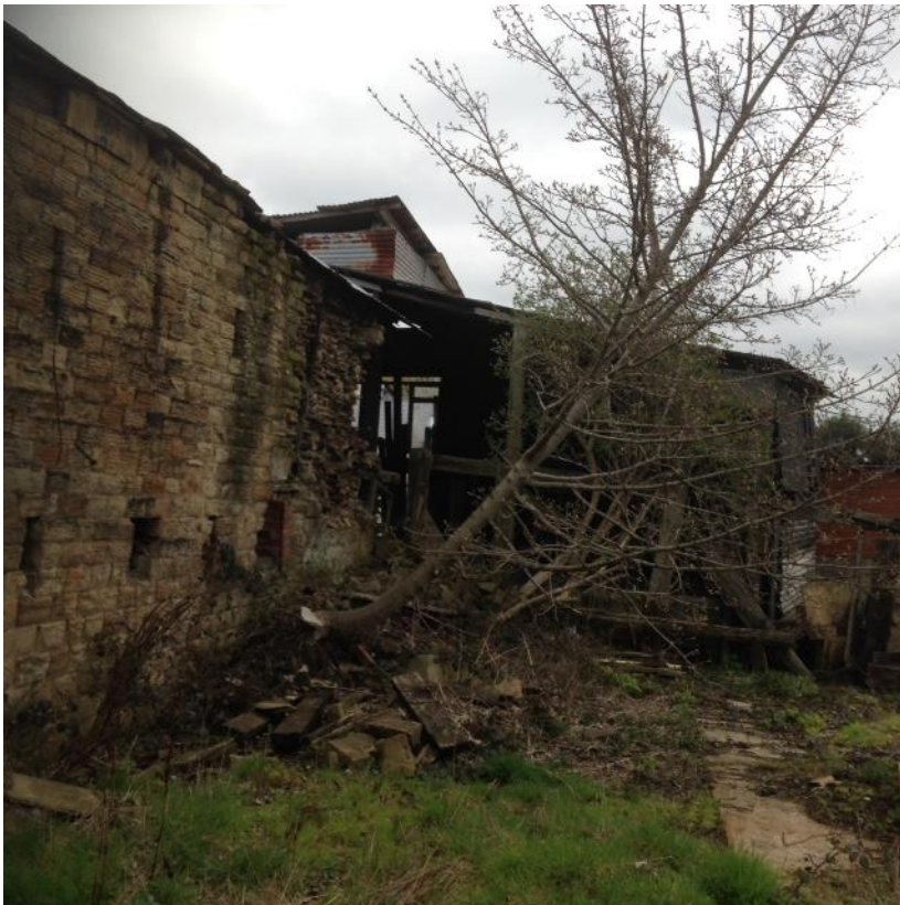
Figure 3- Crumbling farm building structure at Poplar Farm
