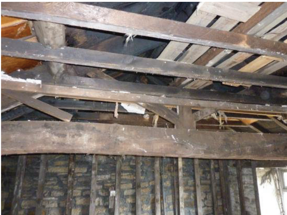
Photo 10: View of fire damage within upper floor of farmhouse.
