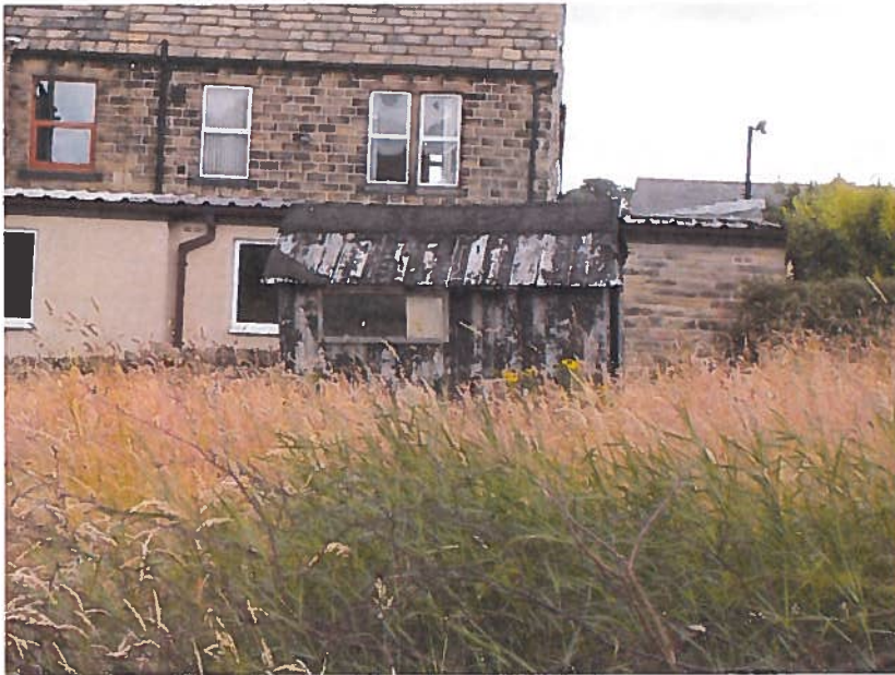
Figure 4: Small dilapidated shed, south east corner.
