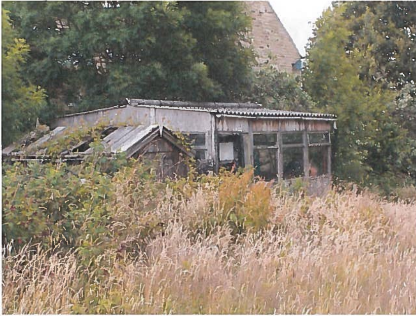
Figure 5: 2 No. dilapidated shed, north west boundary.
