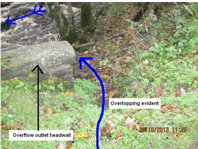
11. Possible overtopping flow path
