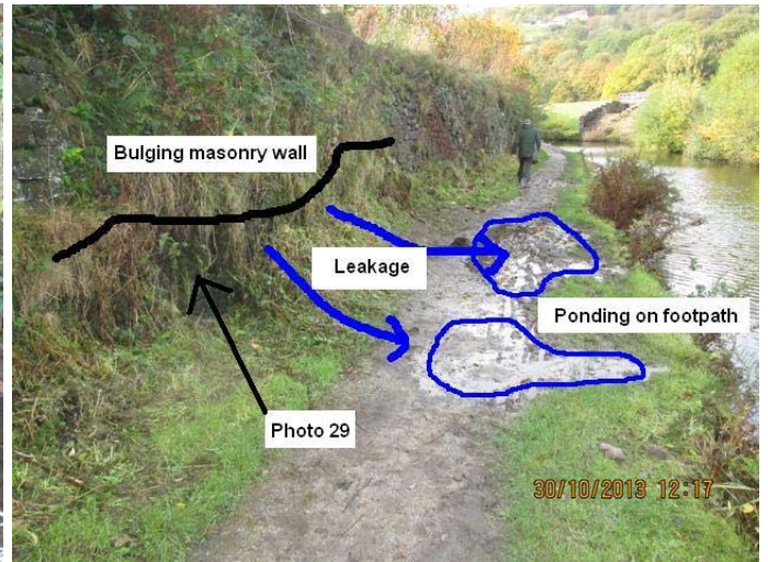
28. Leakage and bulging masonry
