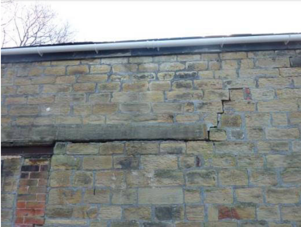
Photo 7: Gaps within stonework (& behind eaves board) on north elevation of Building 2
