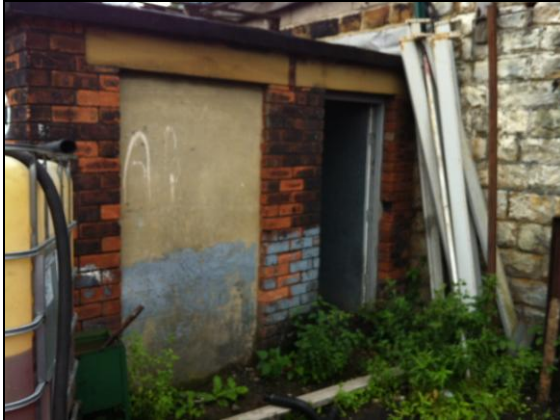
Photo 8 (Electric sub station located NE of site)
