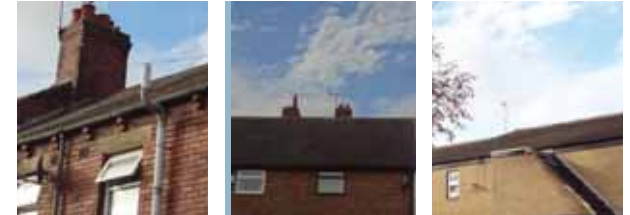
Roofing: High pitched dual tiled roofing on the red brick dwellings. On the Blacker Crescent housing, the pitch is lower and asymmetric
