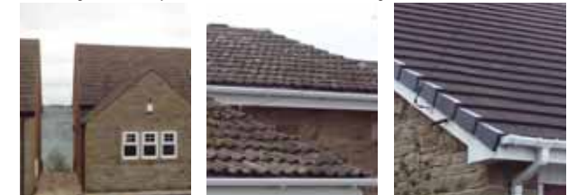
Roofing: A variety of different profiled concrete tiles at low pitch, mainly brown in colour.
