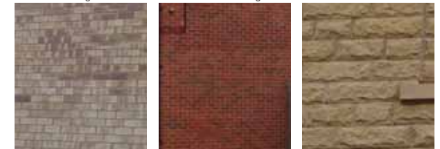
Brick Work: This varies in colour from red to buff with artificial stone
