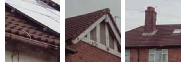
Roofing: Original tiles are profiled red clay pantiles. Gables articulate mid terraces or bookend end units. Some solar panels are in evidence.
