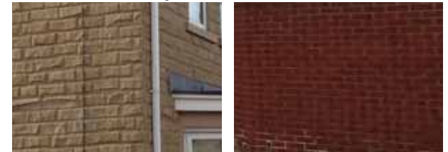
Brick Work: There are 2 main materials, red for the main housing within Olympia Gardens and buff stone for the entrance dwellings
