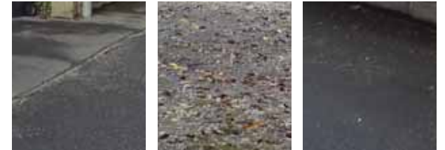
Surface Treatment: The pavements and the roads are made up of tarmac with some gravel driveways.
