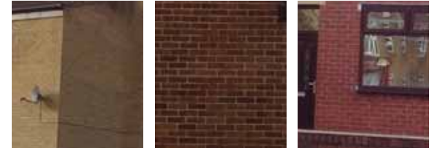
Brick Work: Red/brown bricks are more commonly used apart from the Blackers Crescent housing which is made up of buff bricks
