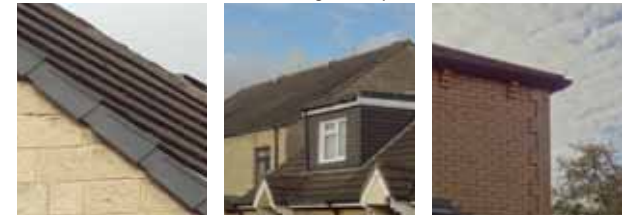
Roofing: It varies in roof pitches and plastic gable end verge materials. The roof tiles themselves appear to be concrete or natural slate
