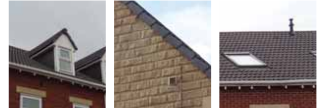
Roofing: Standard modern roofing materials with plastic gable end verge materials and no chimneys
