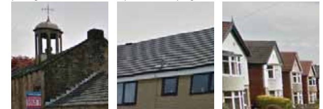
Roofing: Standard modern roofing materials with plastic gable end verge materials and no chimneys
