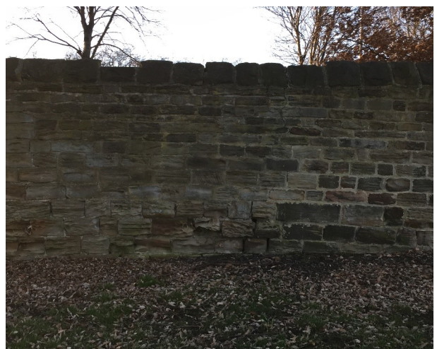
Figure 8 - View of the erosion to the boundary wall with newer section of stonework to the right
