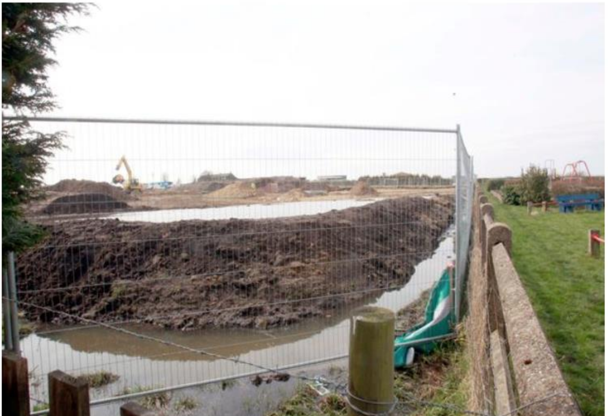
The groundworks site for new homes in Scholes which has caused flooding in to Hazel's garden and the children's play area behind her home
