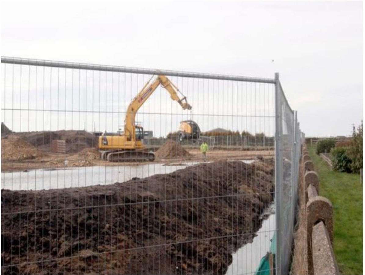
The groundworks site for new homes in Scholes which has caused flooding in to Hazel's garden and the children's play area behind her home
