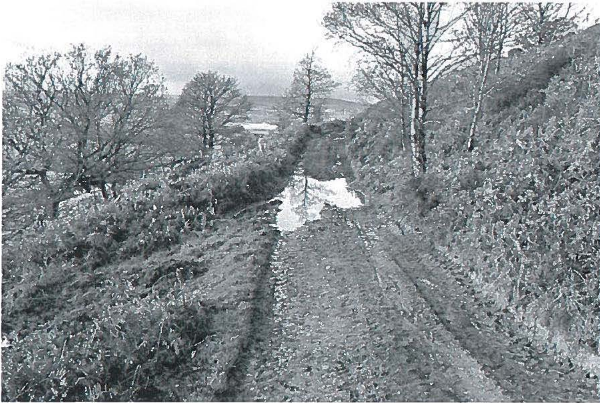
Photo below shows drainage issue and braken.
