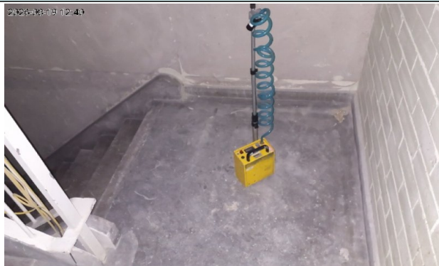
Sampling pump (sample ref: 26/8/A/19/MH12)
