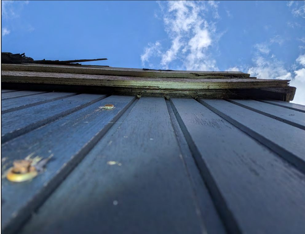
Plate 4: Gap behind fascia board on N, W and S elevations of B2, but well-sealed.
