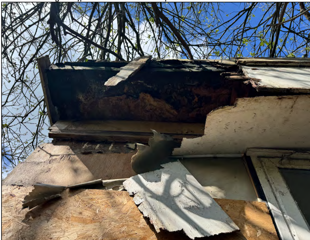
Plate 7: Damaged soffit on eastern elevation of B2.
