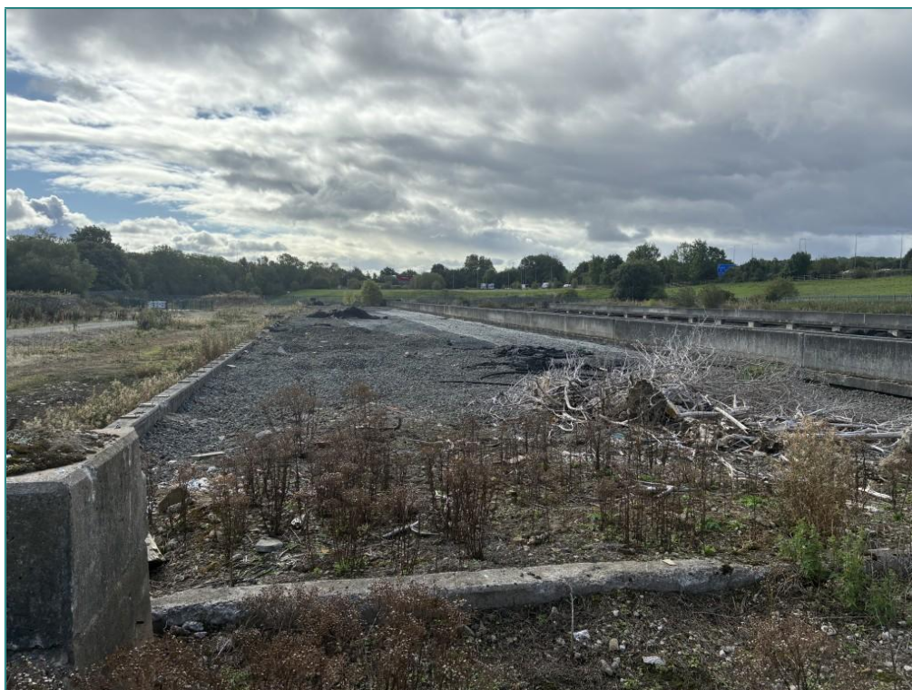
Photograph 2: View Looking South at One of the Full Filter Bed.
