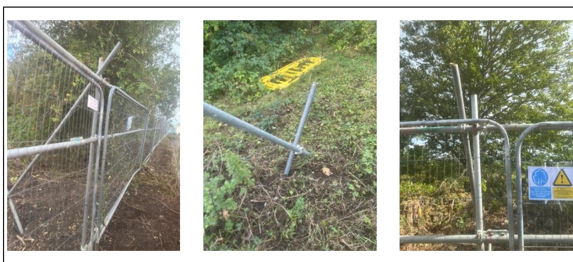
Figure 4.1: Examples of BS5837:2012 compliant scaffold framework temporary tree protection barriers.
