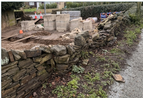
Photo 5 - 16 March 2026. A substantial length is damaged or dismantled, with natural stone displaced into irregular piles.
