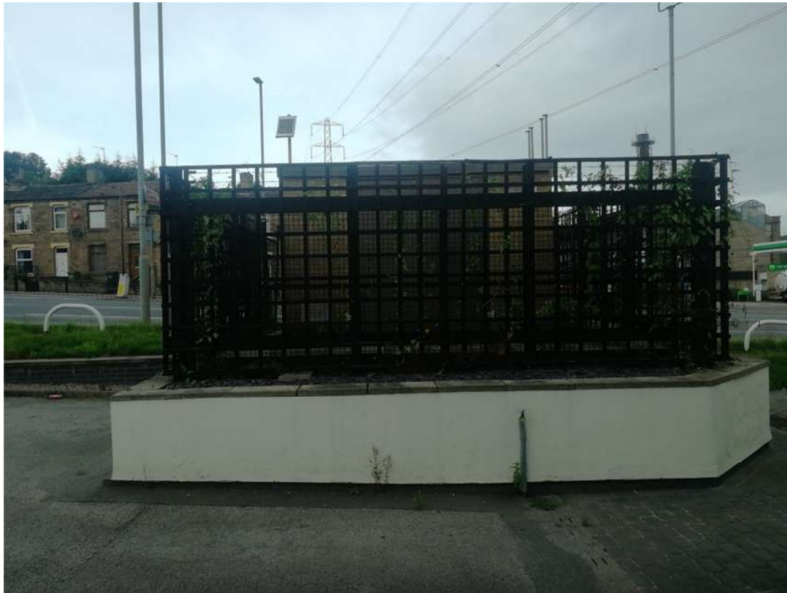
Photograph 22: Gas governor at northwest boundary of site (off site).
