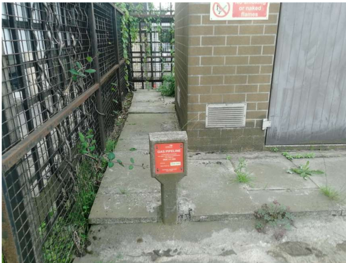
Photograph 22: Gas governor at northwest boundary of site (off site).
