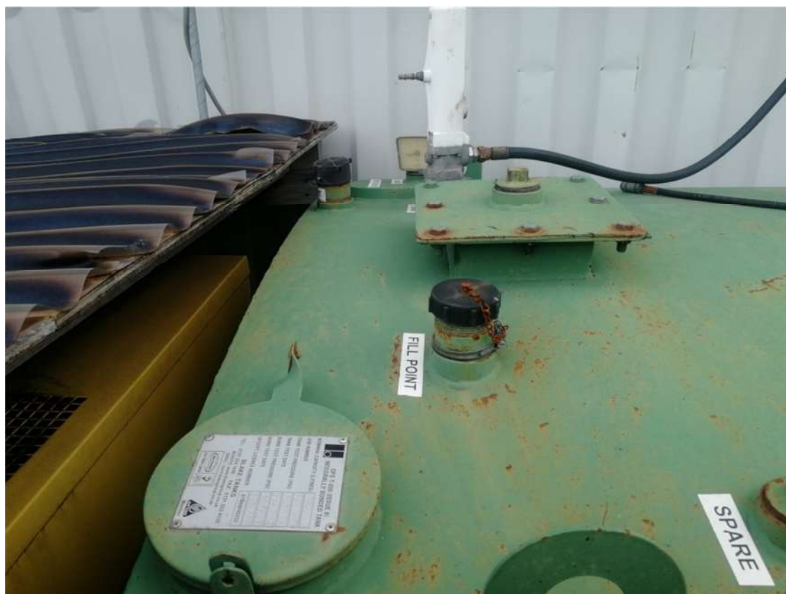
Photograph 12: Above ground oil storage tanks at southwest corner of main building.
