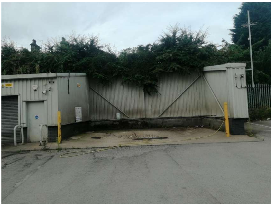
Photograph 18: Drain for car wash at the western boundary, facing west.
