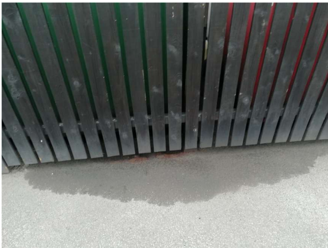
Photograph 13: Potential oil staining beneath above ground oil storage tanks.
