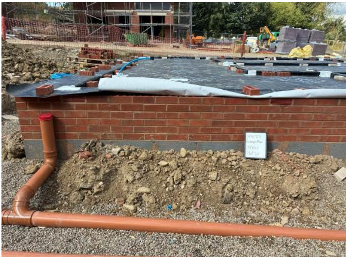
Photograph 14: View of evenly spaced periscopic vents on Plot 20. 19/8/26
