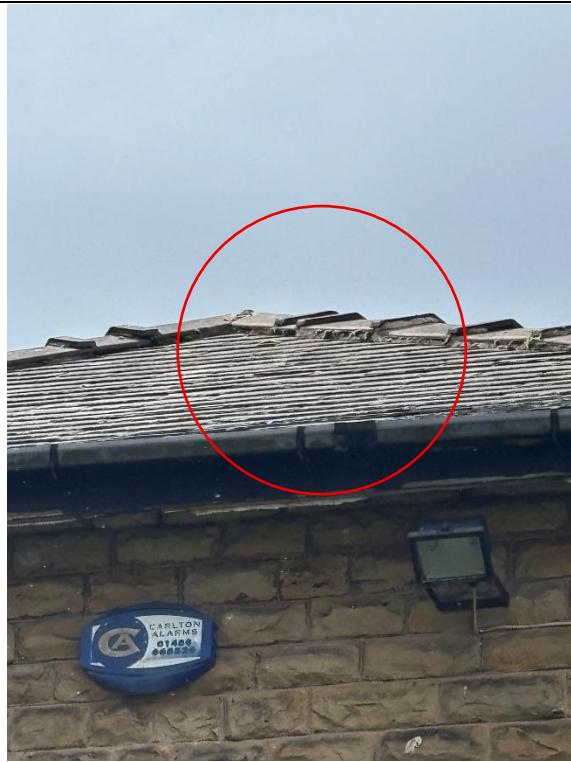
Photograph 14: View of the dislodged roof tiles on north facing elevation.
