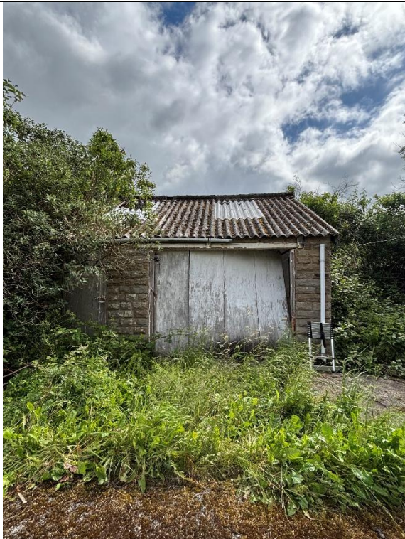
Photograph 7: View of the garage building. Poor condition doorway.
