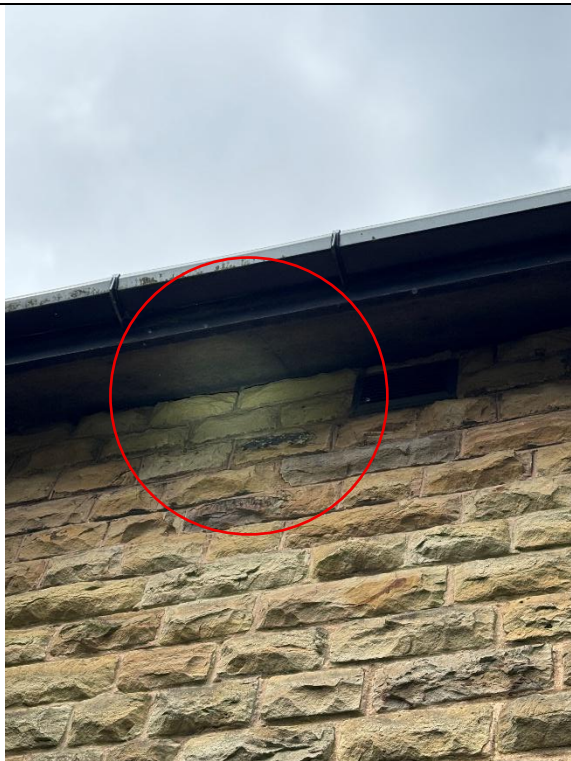
Photograph 15: View of the localised gaps where eaves meet the wall plate.
