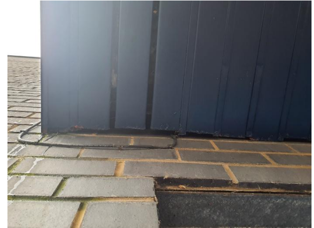
Gap beneath overhanging balcony of B1
