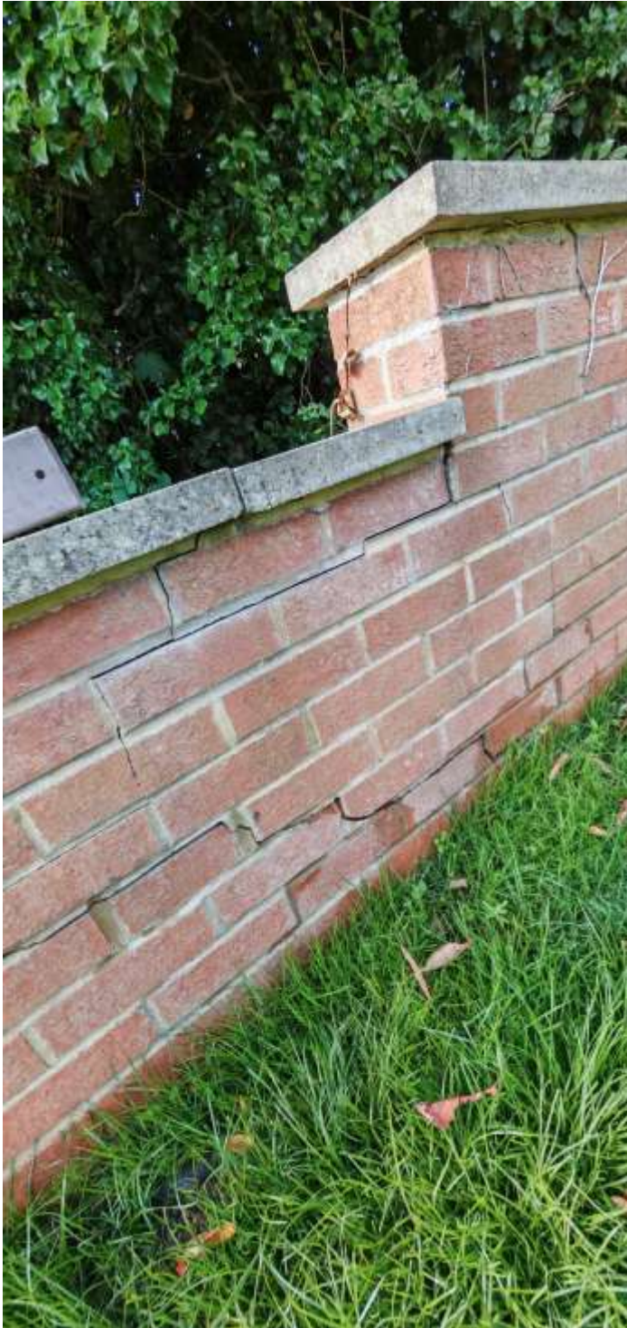
Image of crack to small boundary wall
