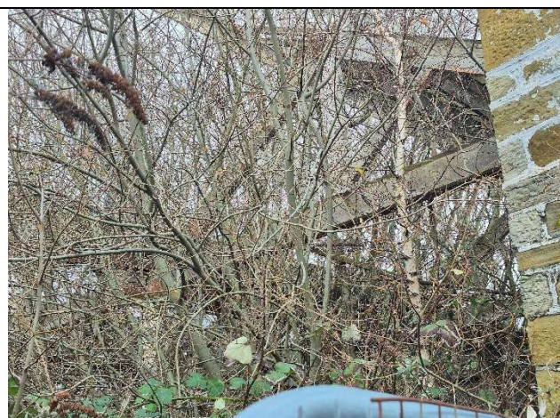
Photo 13: woodland two within derelict building at southeast of site.
