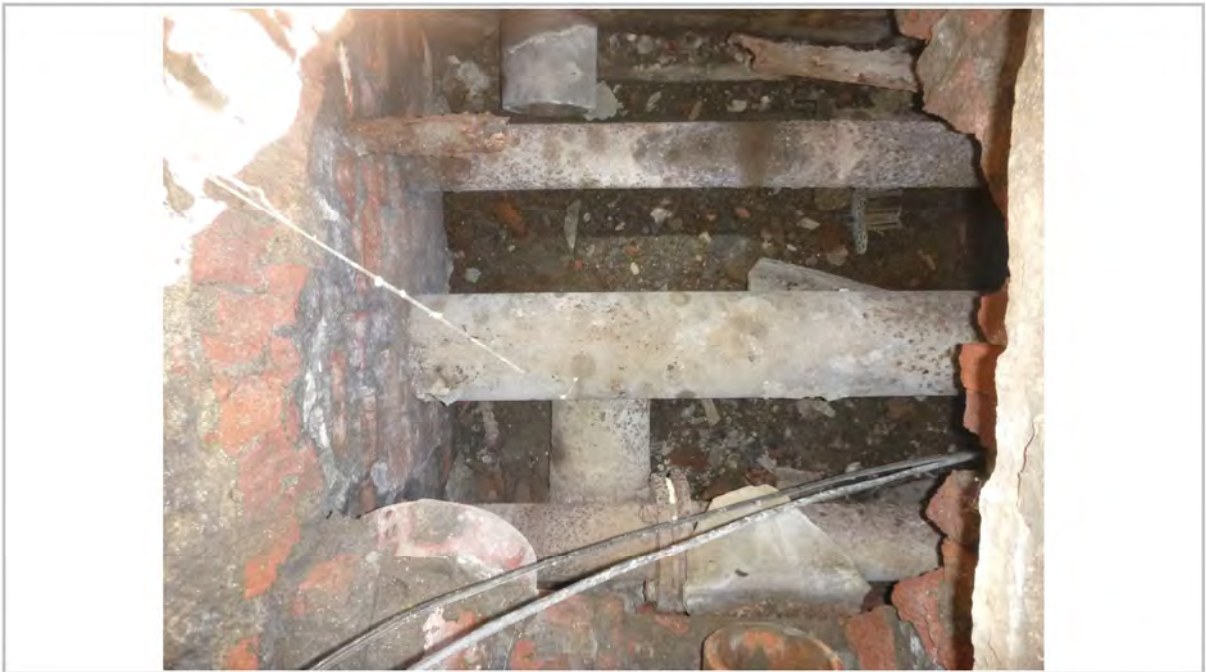
GP25 SERVICE DUCT
