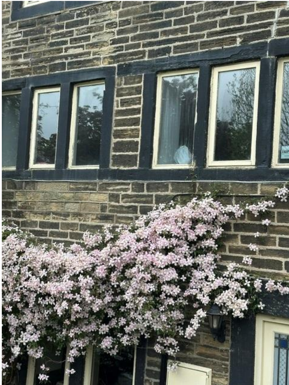
Photograph showing rear elevation window condition
