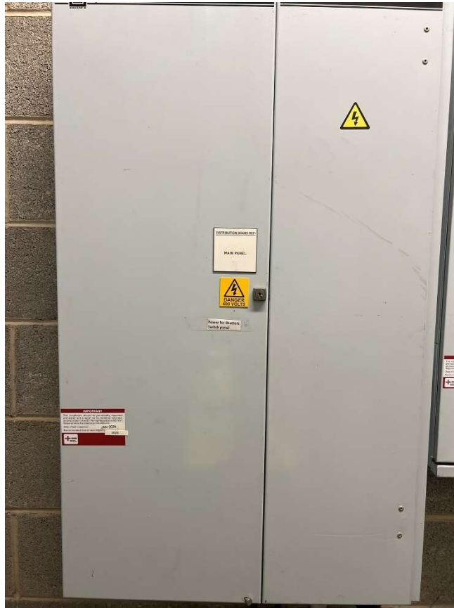
Existing Main Panel Board – Located within Main Switch Room
