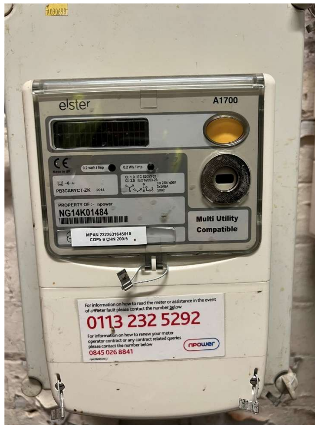
Existing Incoming DNO Meter – Located within Main Switch Room
