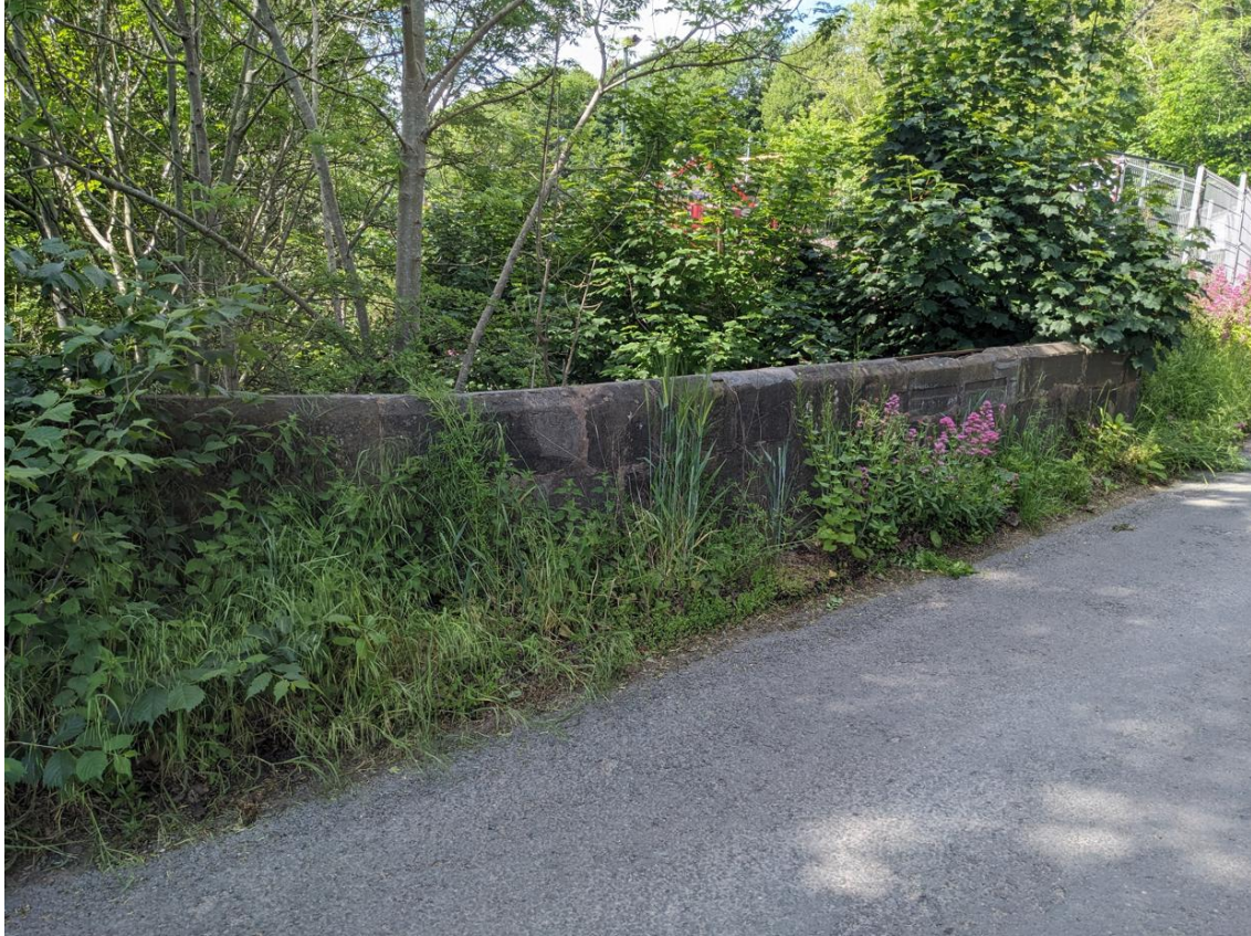
Photograph 25 - General View Along North Parapet And Verge with increased Vegetation
