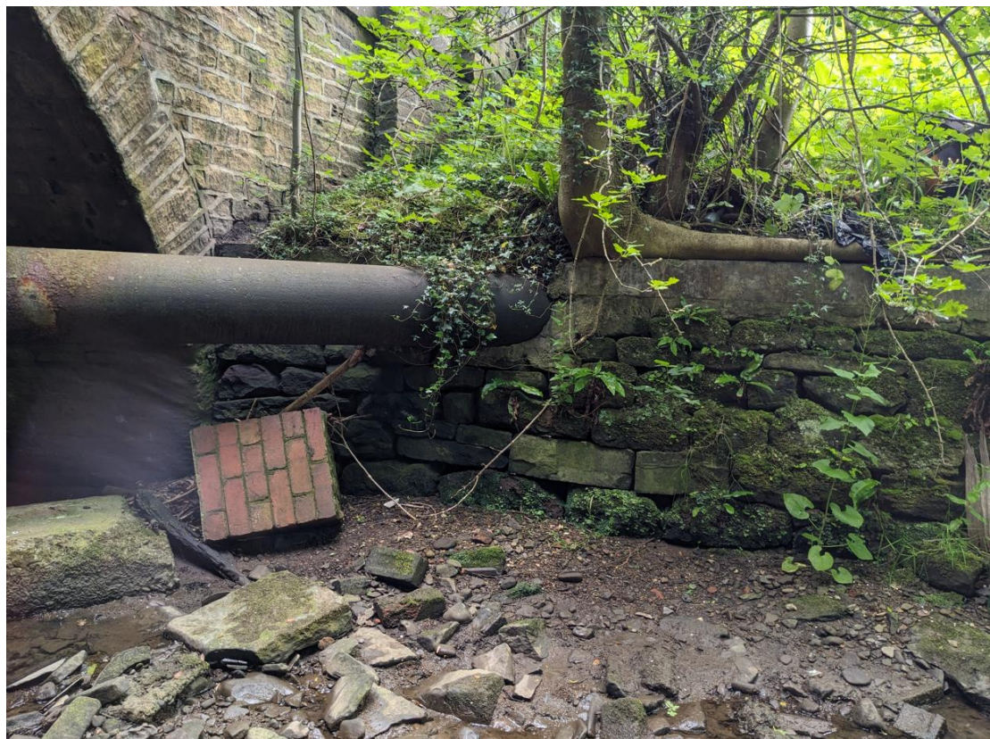
Photograph 14 - Failed Support To Service Pipe, Downstream
