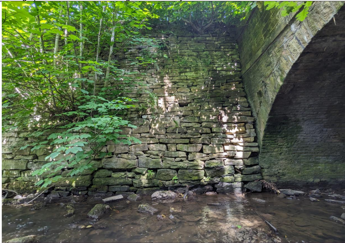
Photograph 22 - North East Training Wall Exhibiting Bulging And Established Sapling Growth
