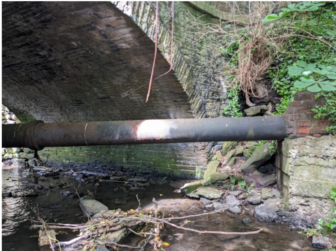
Photograph 13 - Failed Support To Service Pipe, Upstream
