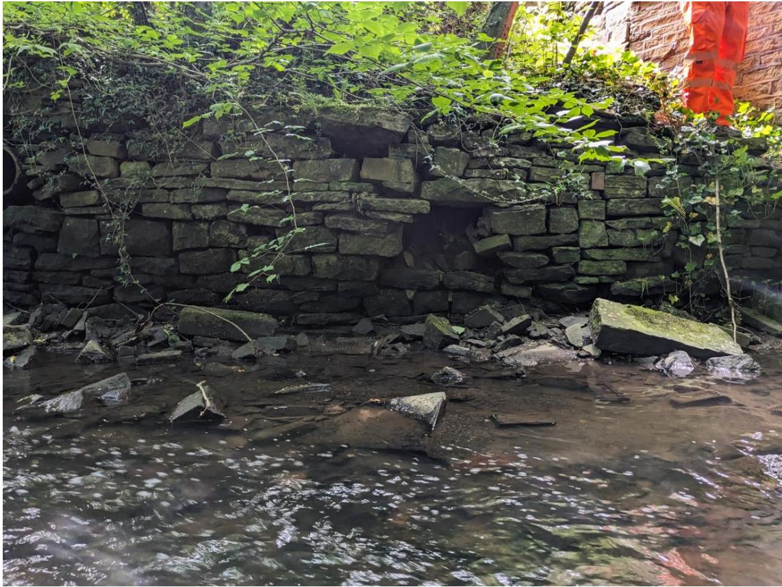
Photograph 19 - South West Training Wall Exhibiting Partial Collapse Due To Established Tree Growth, Increased Deterioration Since 2025 Principal Inspection
