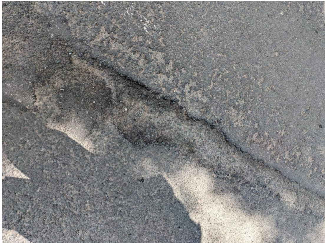
Photograph 29 – 1.5m By 150mm Wide Rutting To Centreline Of Carriageway, West End Of Structure
