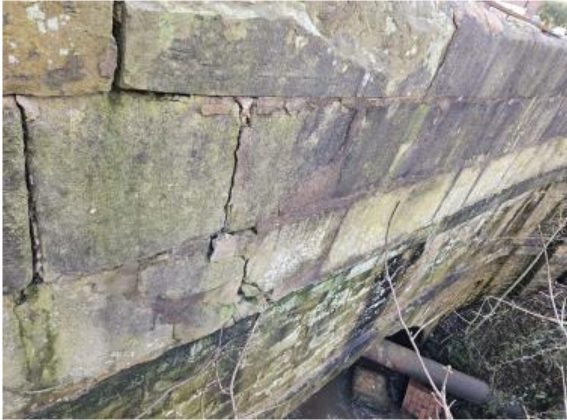
Photograph 23 – Cracking Through Mortar To North Parapet At East End, Full Height, Open 5-10mm
