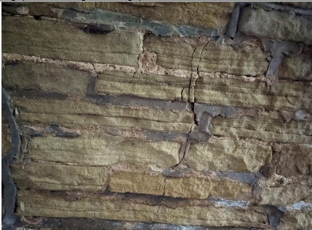
Photograph 32 – 0.5m Length Cracking Open 1-2mm Through Mortar And Masonry To west \frac{1}{4} Point, Midway Along Structure Width
