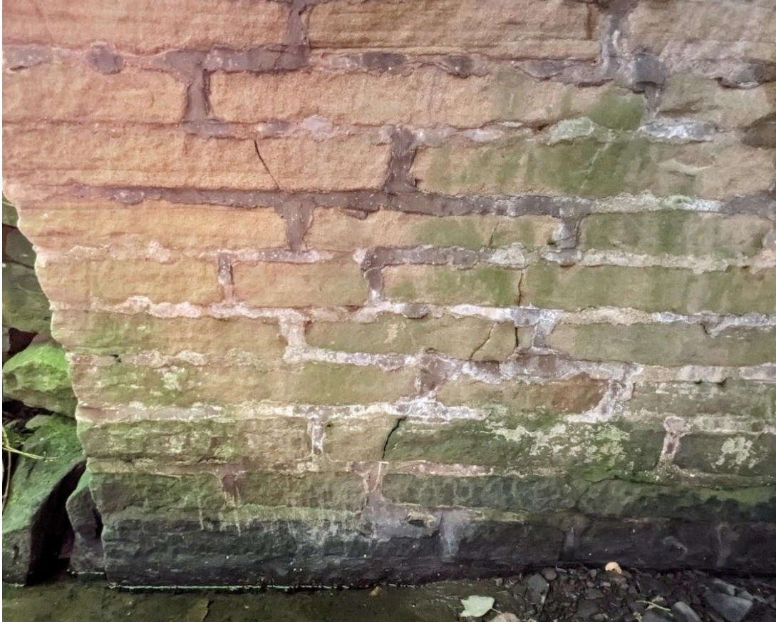
Photograph 31 – 0.5m diagonal cracking open 1-2mm to south end of structure below west \frac{1}{4} point
