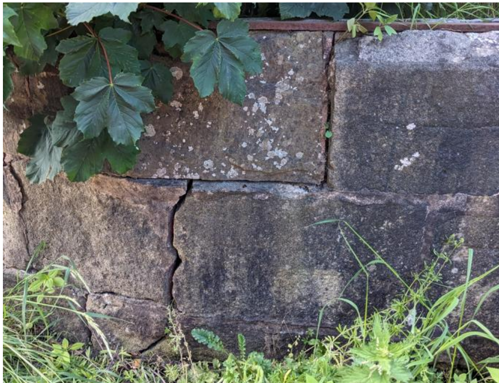
Photograph 24 - Cracking To North Parapet Through Masonry, East End, Full Height, Open 5-10mm
