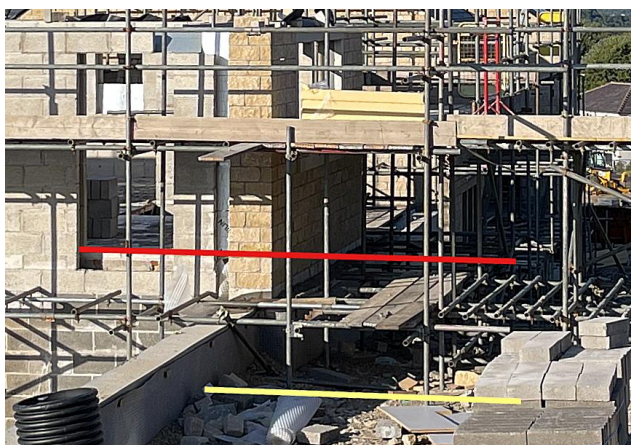
Plot 23, Lingards Fold Red line: Ground floor level – doorway leading into yet to be constructed garage Yellow line: Apparent garage threshold level
