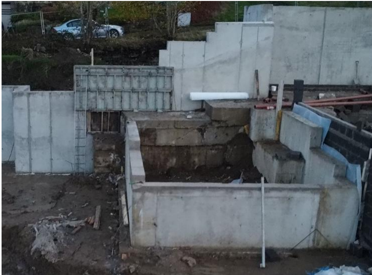
Illustration B Plot 23 – Unexplained foundations
