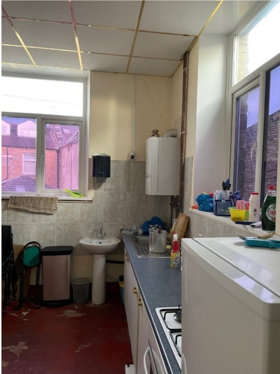
Figure 6: Adjacent kitchen showing the window facing into the extension zone (right of image), which will be superseded by the proposed works.
