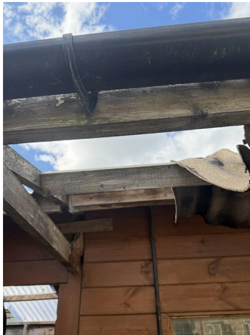
Photograph 4 — Eaves detail: degraded, torn roofing membrane and open gaps to the sky at the roof edge.
