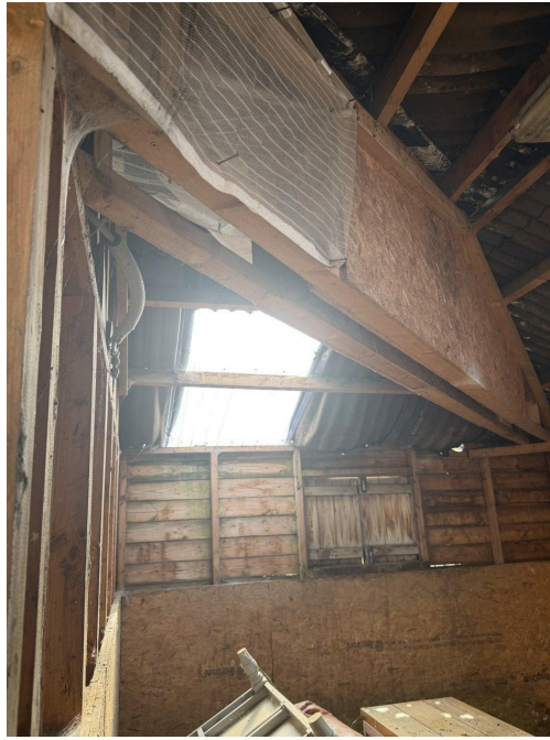
Photograph 3 — Internal view: open underside of roof with torn lining, daylight ingress through gaps and extensive intact cobwebbing.
