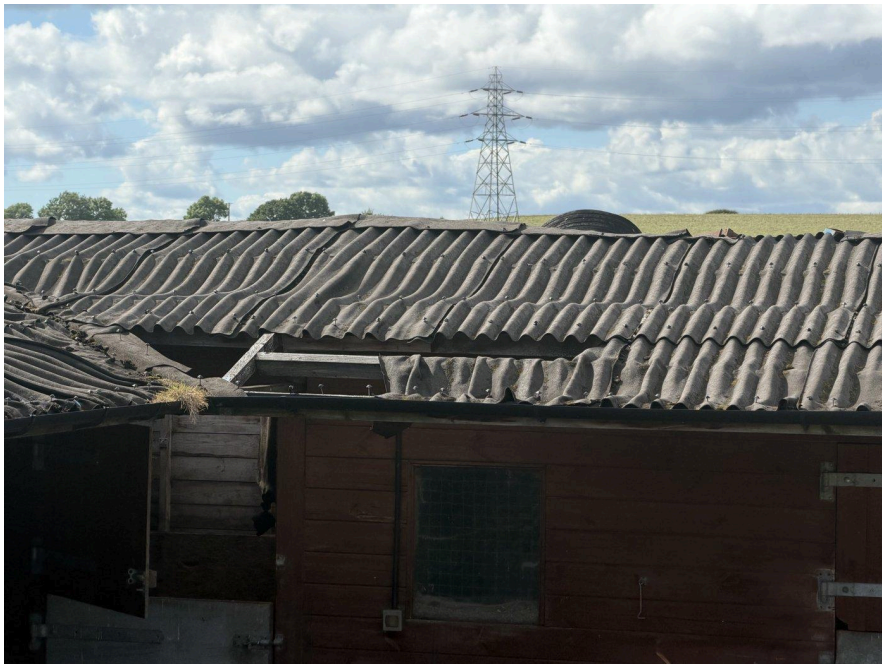
Photograph 2 — Roof condition: weathered and locally displaced fibre-cement sheets; open, lightweight timber structure.
