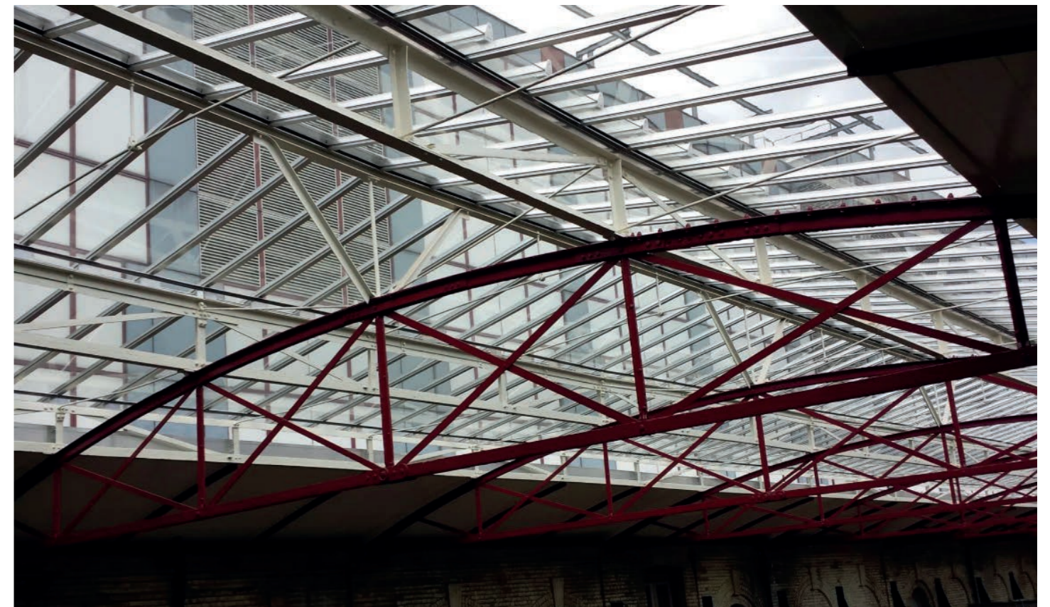
Fig 4.1.2 Farringdon Rail Station illustrating the 'Traditional' capped glazing system - same as proposed
