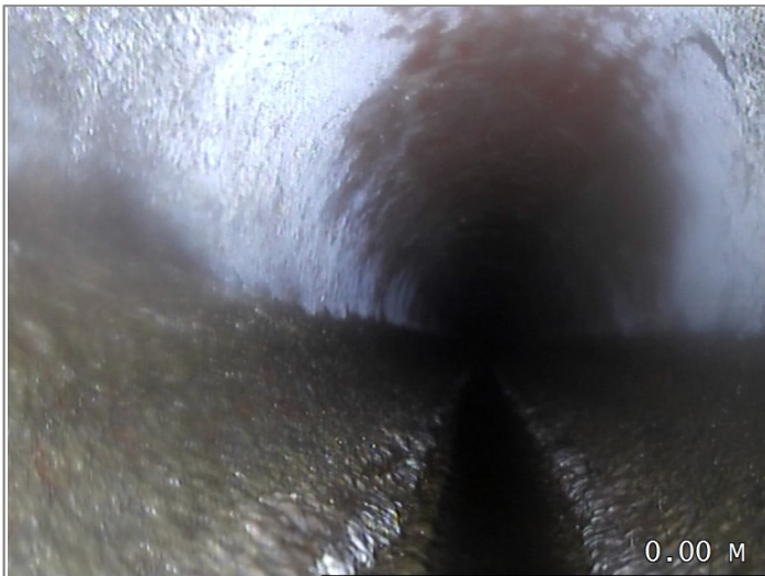
Start node type, manhole, reference MH 5 B2
