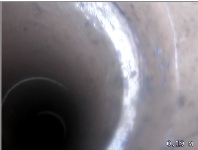
Start node type, manhole, reference MH2 B1
