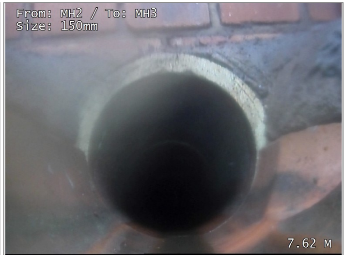
Finish node type, manhole, reference MH3
