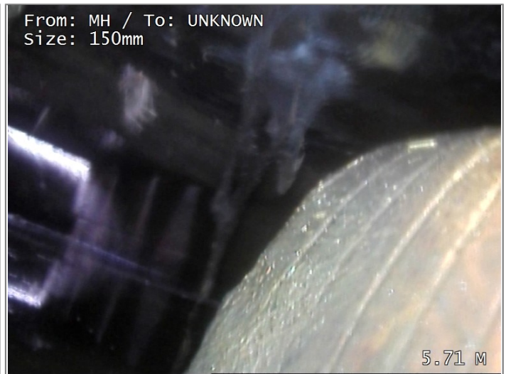
Finish node type, other special chamber, reference CESSPIT WHICH PUMPS TO SLURRY TANK
