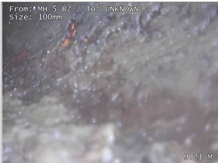
Line of drain/sewer deviates left
