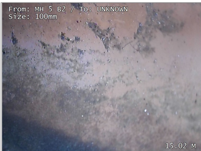
Line of drain/sewer deviates left
