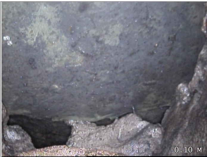
Start node type, manhole, reference MH 1 B3
