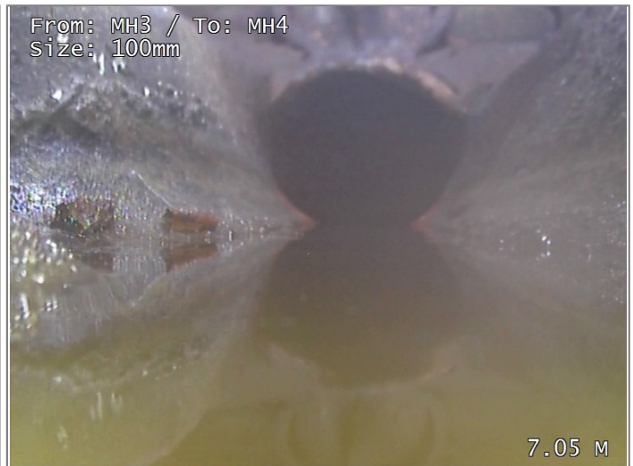
Finish node type, manhole, reference MH4
