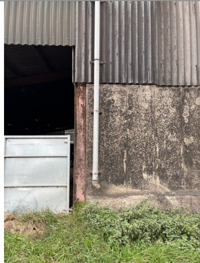
Other Site Photos: RW pipe on to ground
