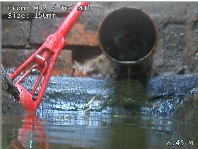
Finish node type, manhole, reference MH1
