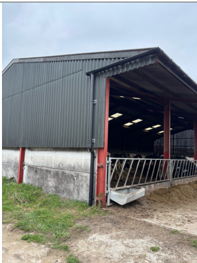
Other Site Photos: RW pipe on to ground
