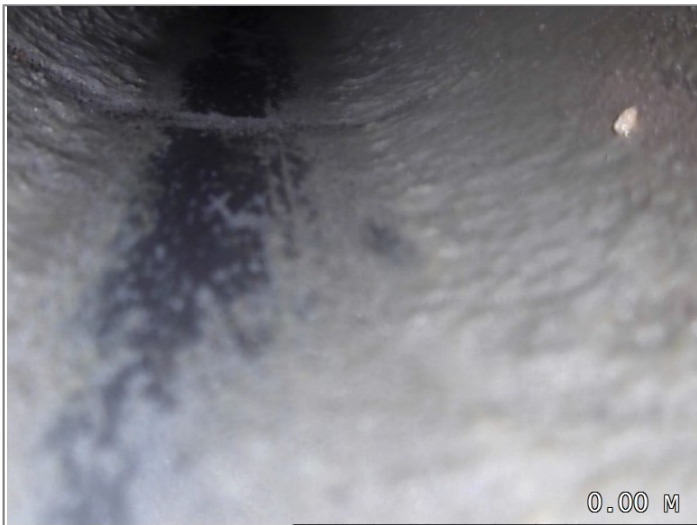
Start node type, manhole, reference MH5
