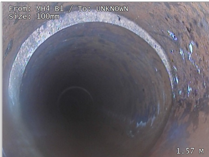
Joint displaced medium
