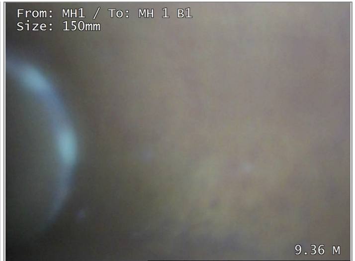
Line of drain/sewer deviates left
